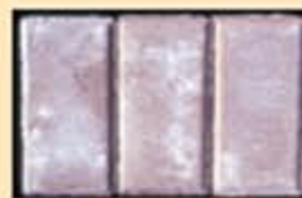
Pavers with efflorescence.
